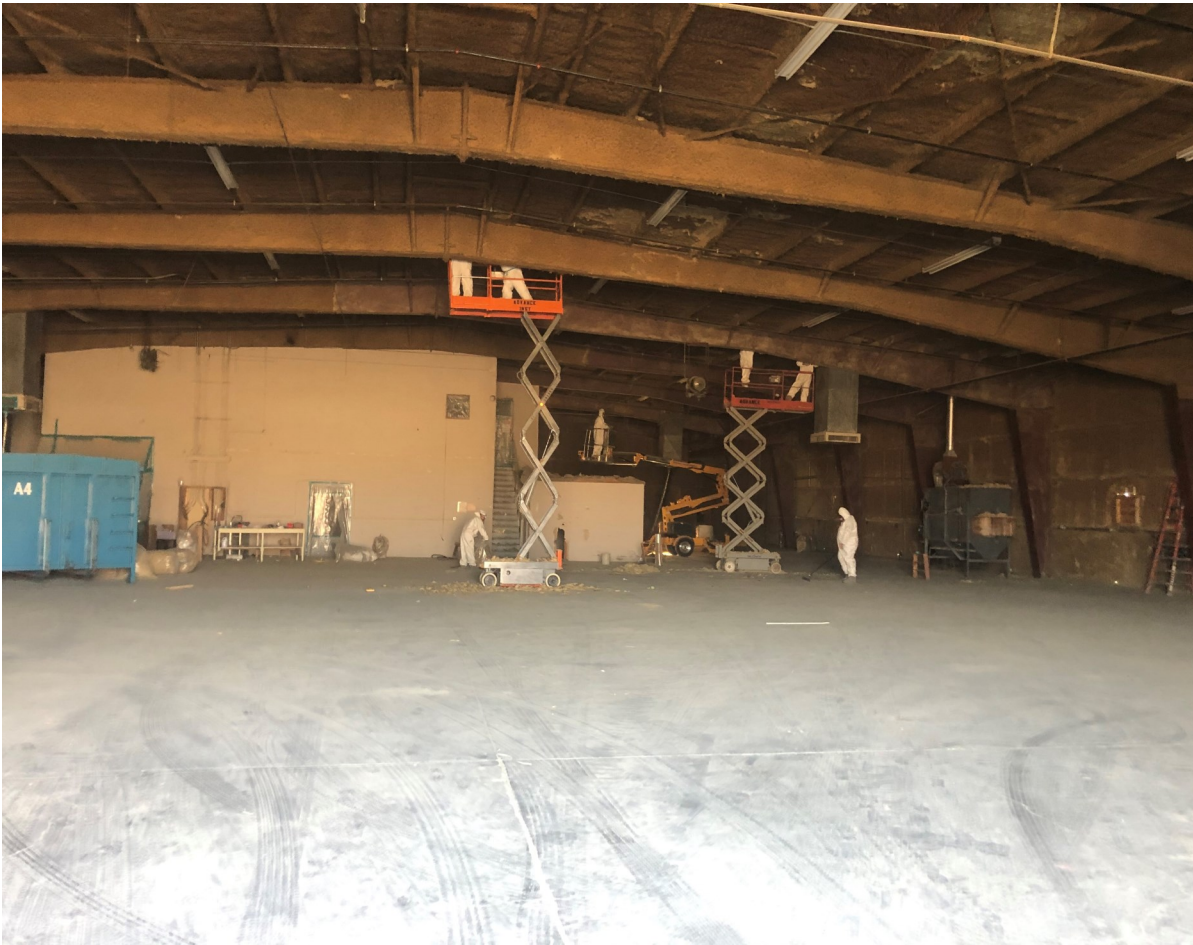
Early work of converting the NEVCO building in Wadsworth to a food bank
